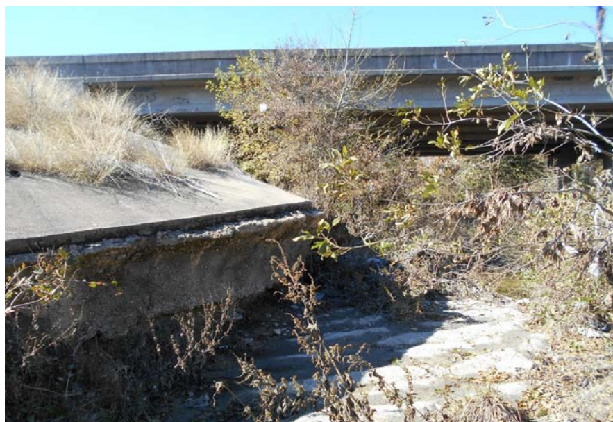
The downstream bridge abutment for the Roy Reynolds Bridge. Nolan Creek is eroding/undermining the concrete abutment.
