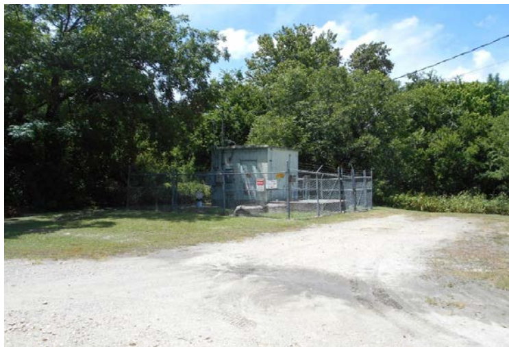
VFW Lift Station Wetwell
