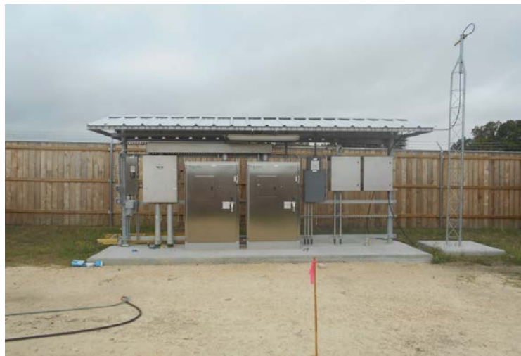
Rummel Lift Station
