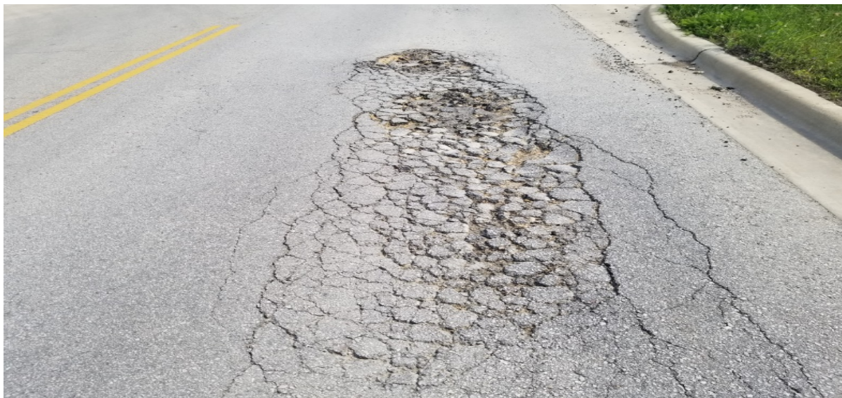
One example of damage done by Winter Storm Uri.
