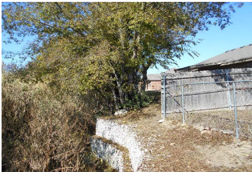
Part of the current erosion out of the City's drainage easement.
